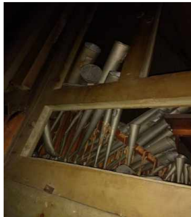
ABOVE: IN THE SOLO DIVISION, THE RACKING THAT SUPPORTED THE 8' TUBA SEEMS TO HAVE FAILED, CAUSING THE PIPES TO COLLAPSE UNDER THEIR OWN WEIGHT.
